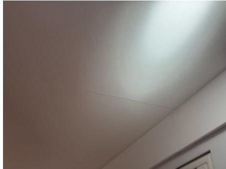
Ceiling cracking was observed, the installation of an expansion joint will reduce the likelihood of this recurring once repaired.
