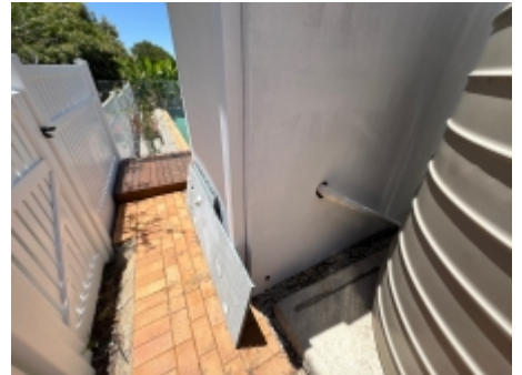
A 75 mm exposed slab edge should be maintained under all external cladding. a pest controller should be engaged for further advice.
