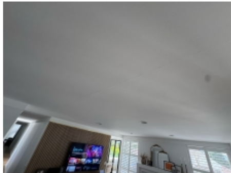
Ceiling cracking was observed, the installation of an expansion joint will reduce the likelihood of this recurring once repaired.
