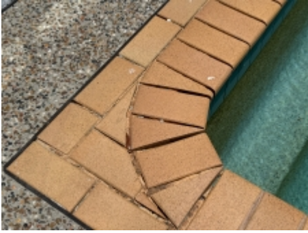
Pool coping pavers require re-grouting.
