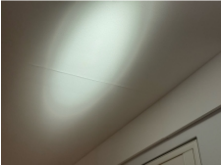
Ceiling cracking was observed, the installation of an expansion joint will reduce the likelihood of this recurring once repaired.
