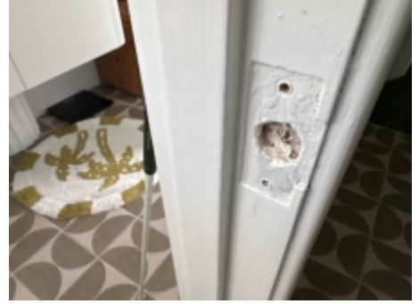
Patching and painting is required.
