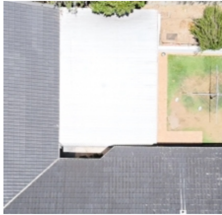
Corroded screws will eventually cause rust on the roofing iron, leading to water ingress. A licensed roofing contractor should be consulted for further assessment.
