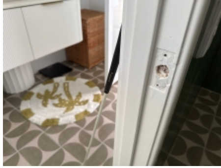
Patching and painting is required.
