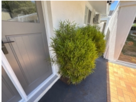
Gardens up against the house hinder the visual inspection zone's, hard surfaces abutting the building are always recommended. A pest controller should be engaged for further assessment.
