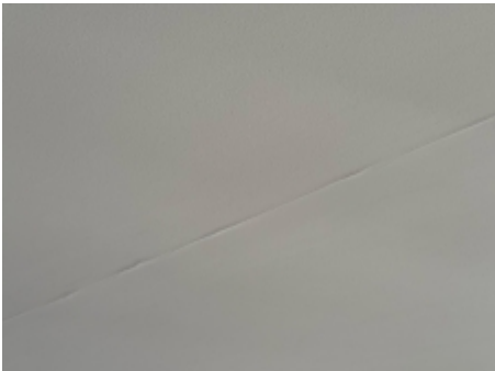
Ceiling cracking was observed, the installation of an expansion joint will reduce the likelihood of this recurring once repaired.
