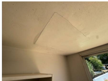
Evidence of previous water ingress at the rear of the garage was observed, moisture testing was performed and no elevated levels were detected.
