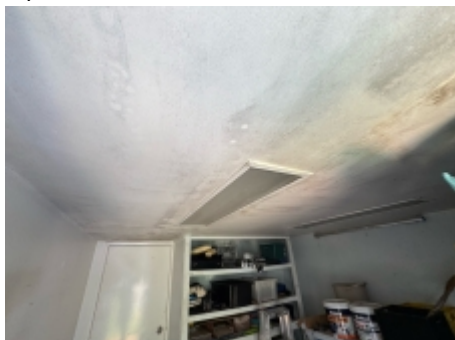
Evidence of previous water ingress at the rear of the garage was observed, moisture testing was performed and no elevated levels were detected.
