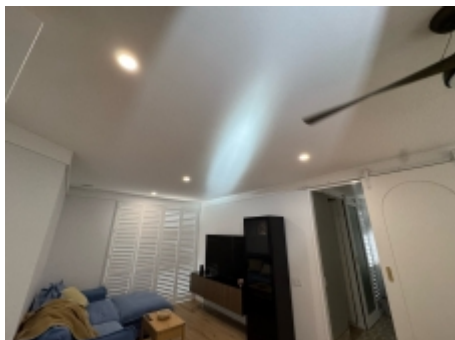
Ceiling cracking was observed, the installation of an expansion joint will reduce the likelihood of this recurring once repaired.
