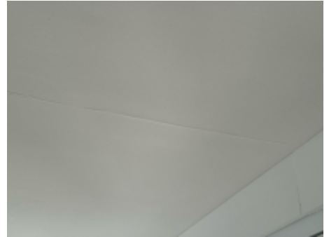
Ceiling cracking was observed, the installation of an expansion joint will reduce the likelihood of this recurring once repaired.
