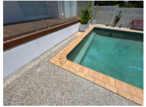
Pool coping pavers require re-grouting.
