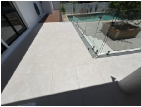
Drummy tiles were observed, resin injection may be a suitable repair.
