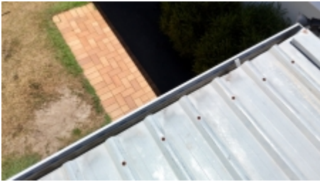
Corroded screws will eventually cause rust on the roofing iron, leading to water ingress. A licensed roofing contractor should be consulted for further assessment.
