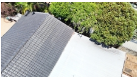
Foliage needs to be cleared away from all structures and debris needs to be cleared out of gutters.
