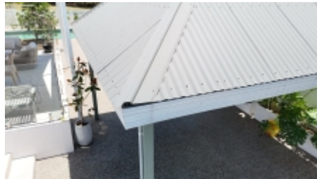
Rainwater goods have not been installed to the gazebo.
