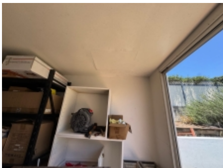
Evidence of previous water ingress at the rear of the garage was observed, moisture testing was performed and no elevated levels were detected.
